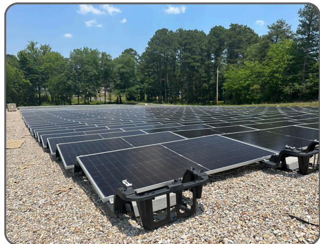
Hot Springs, AK 390 kW (Gravel)
